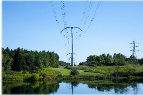
345kV BOLD Double-circuit (3-conductor)
